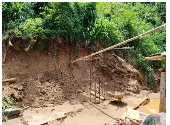
Figure 4h: At the failed bottom of the steep slope location 02 (L2)
