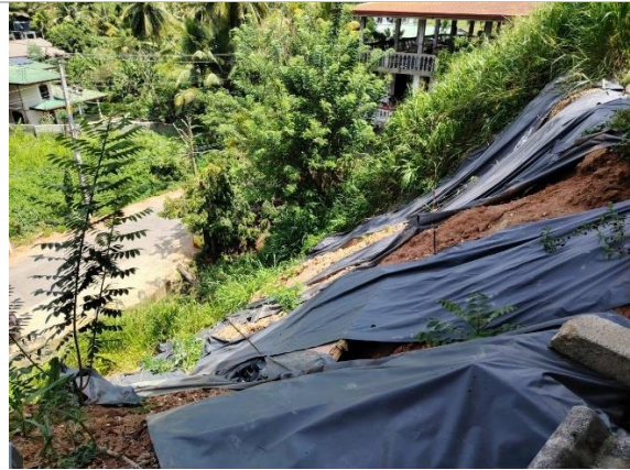
Figure 4b: Tarpaulin covered failure steep slope in between Mahindodaya laboratory and Kiribathkumbura–Wathurakumbura road (Location 01 (L1))
