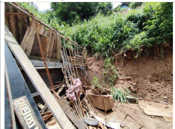
Figure 4i: Destructed retaining wall and property of the resident adjacent house at location 02 (L2)
