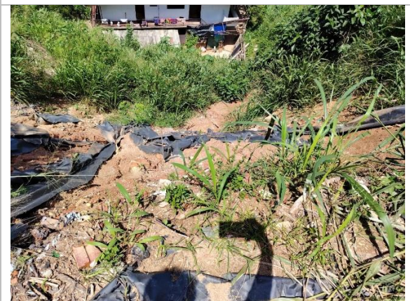
Figure 4g: Steep failed downslope at location 02 with covered by Tarpaulin and nearby house at the toe area of the slope
