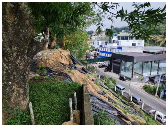
Figure 4c: Destroyed retaining wall at the edge of the upslope with rock (Location 1) Kandy - Jaffna main road (A9) is observed at the downslope
