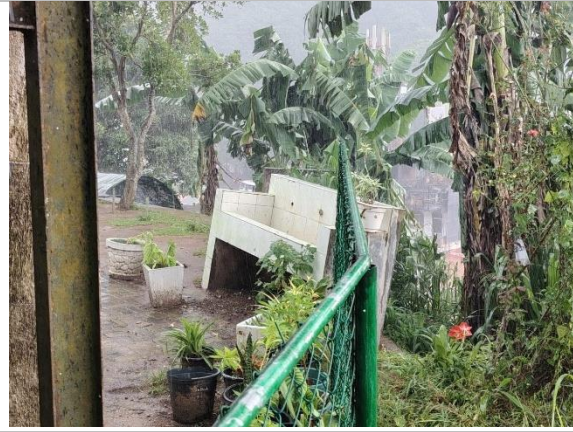
Figure 4e: Abandoned washing basin, risk slope, and vegetation (Location 2)
