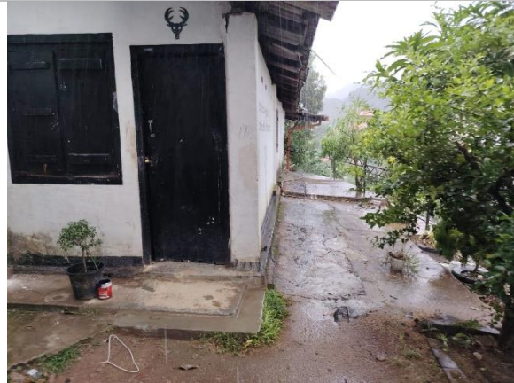
Figure 4l: Single-storey canteen building beside the cadet band building with cracked walls (Location 3)
