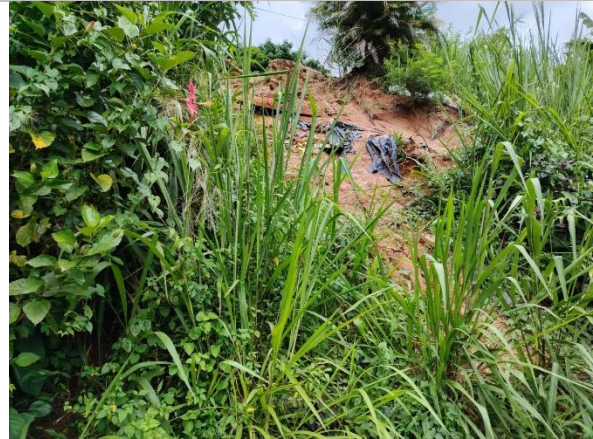
Figure 4b: Location 1; Failed upslope area of the Chapel church
