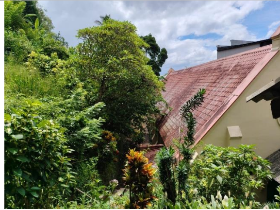
Figure 4a: Location 1; Chapel church and unstable upslope
