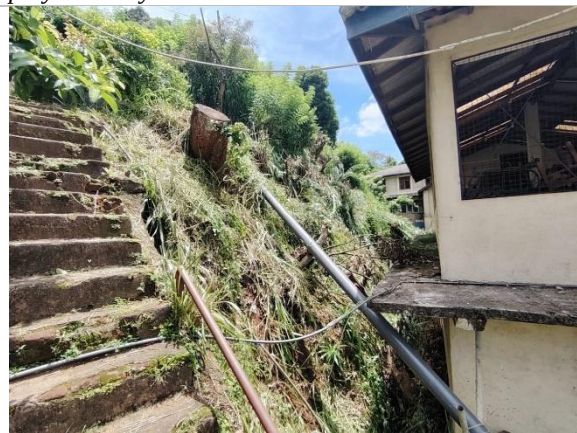
Figure 4e: Location 3; Unstable up slope located behind the school Gymnastic and Karate section
