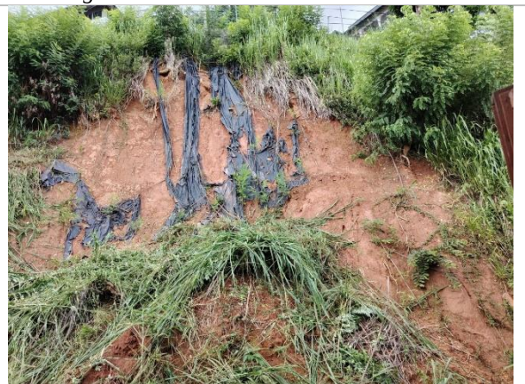
Figure 4f: Location 3; Unstable up slope located behind the school Gymnastic and Karate section
