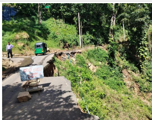
Figure 4a: Location 1; Damaged road and the downslope of the access road
