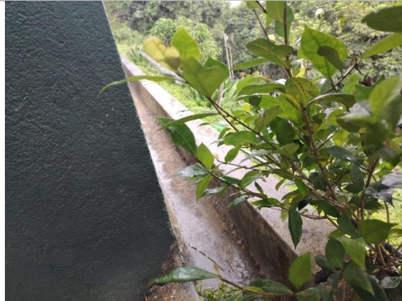
Figure 4k:Location 4; Unstable slope located behind the Grade 8 and 9 classroom building
