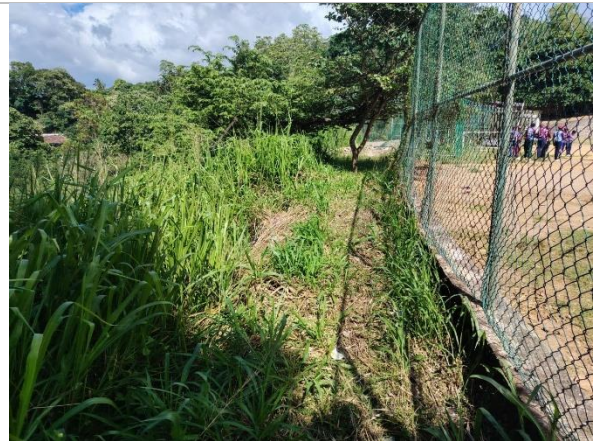
Figure 4f: Location 2; unstable slope behind the cricket practicing net
