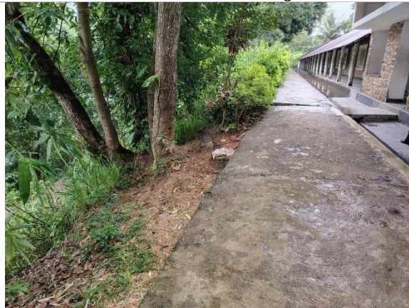
Figure 4m:Location 5; unstable upslope area situated behind the school's aesthetic building
