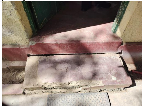
Figure 4h: Location 3 ; Cracks in physical fitness center
