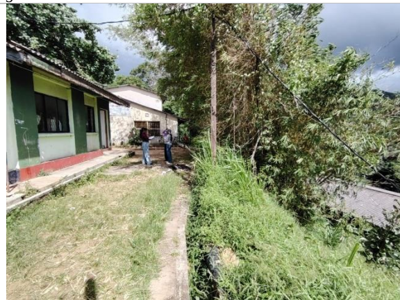
Figure 4g: Location 3 ; failed slope located between the staff room, the physical fitness center
