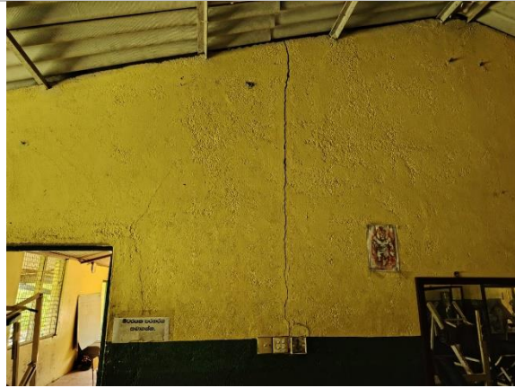
Figure 4i:Location 3; Cracks in physical fitness center wall
