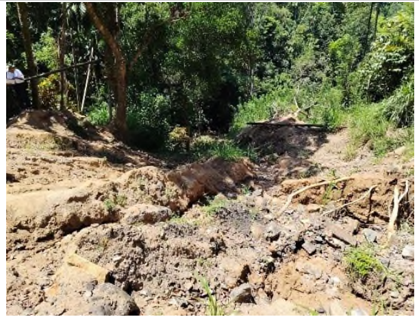
Figure 5f: Vegetation near the landslide of Site No.232, and this area is used as an access road to nearby houses
