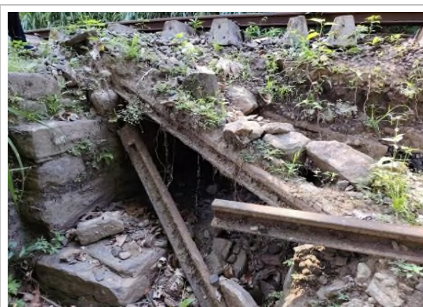
Figure 5b: Seasonal water stream and damaged culvert below the railway line, Site No.231
