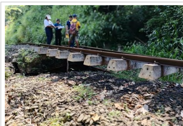
Figure 5a: Vegetation near the washout of the railway line in Site No.231 (CH 60/72)
