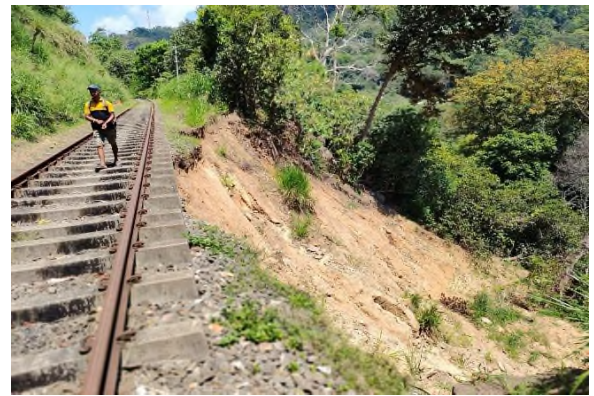
Figure 5l: Damaged downslope section of Site No.235
