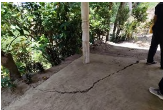
Figure 5m: Cracked floor of high-risk house, Site No.232
