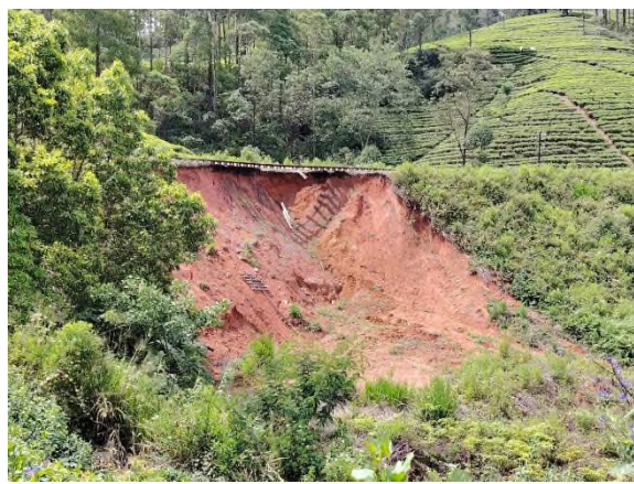
Figure 5a: View of the slope failure and damaged railway crack
