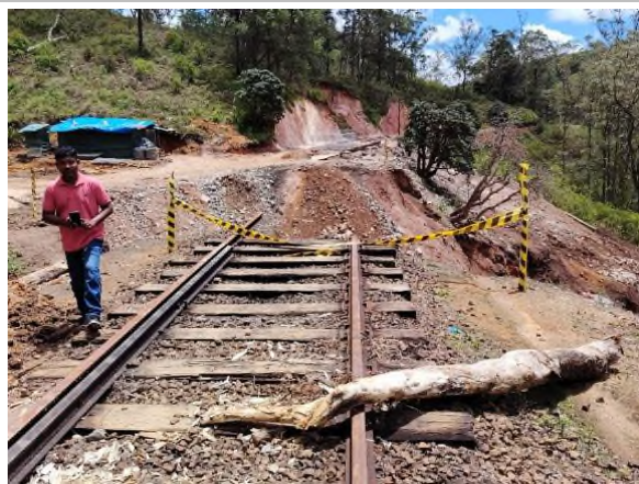
Figure 5a: Washed out railway line from Nanuoya to Ambewela station, Site No: 228 (CH 134/78)
