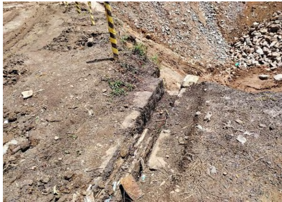
Figure 5g: Culvert nearby location which is blocked with debris
