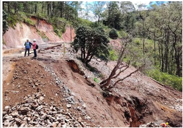
Figure 5f: Steep and cracked slope consisted of Maha-Rathmal
