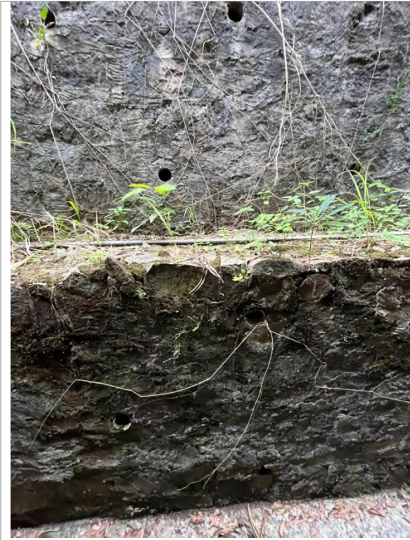
Figure 4g: Crack in the retaining wall
