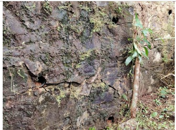
Figure 4j: Cracks in the wall
