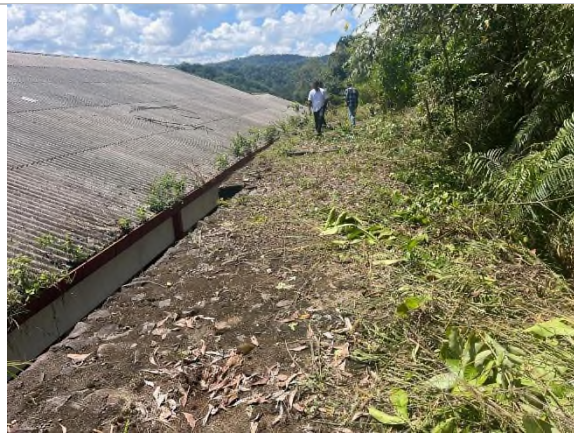
Figure 4c: Upslope view of the unstable area
