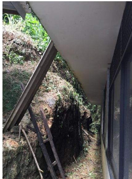
Rock boulders behind the primary school building (Location 03)
