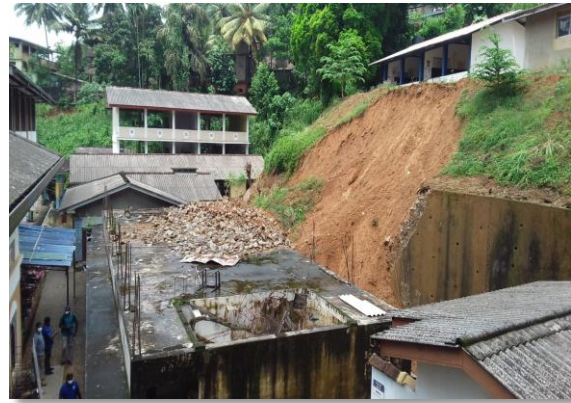
Slope failure occurred in location 01 (behind the main hall)
