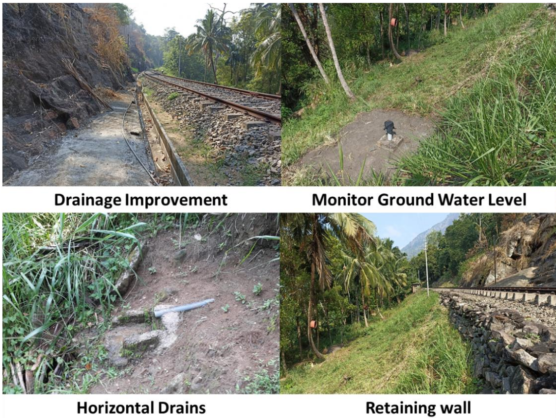
Figure 5 – Remedial measures already undertaken to reduce the potential risk
