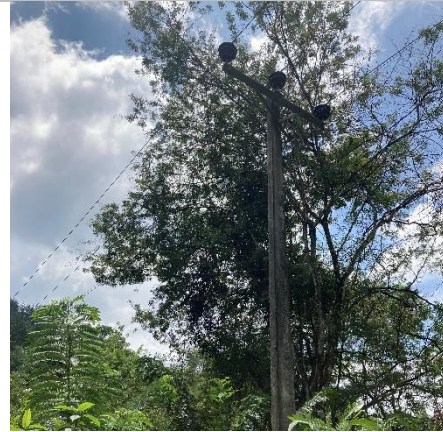
Figure 6b: Electricity supply line of CEB
