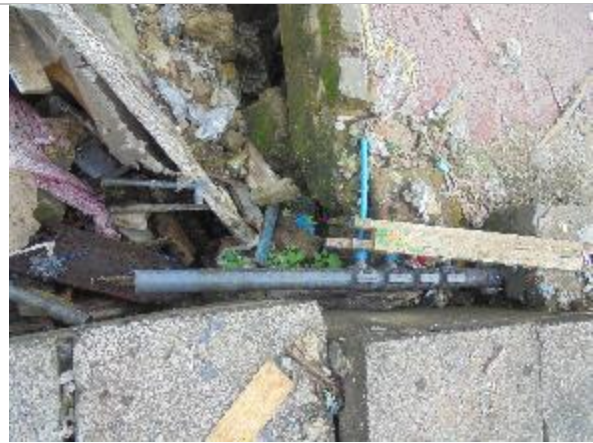
Figure 6d: Water supply lines (already damaged due to the incident)
