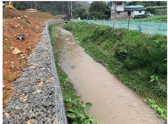
Figure 4h: Stream flowing opposite of the temple (Seetha Eliya Kadura) and existing retaining wall
