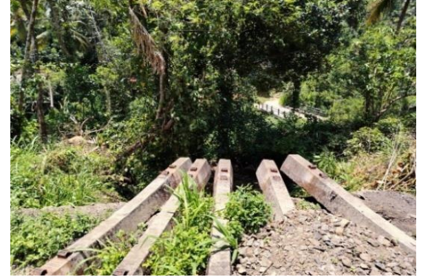
Figure 5j: Vegetation cover along the damaged railway track, Site No.234
