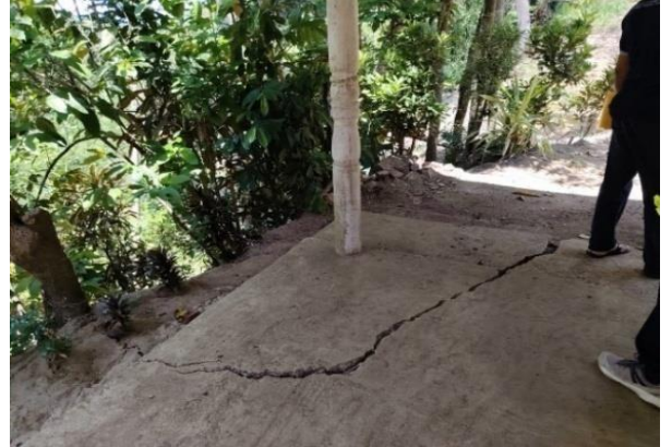
Figure 5f: Cracked floor of high-risk house, Location No.02, Site No.232
