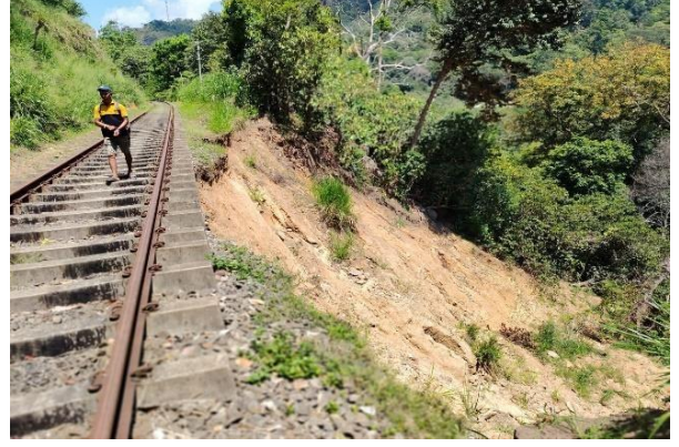
Figure 5l: Damaged downslope section of Site No.235
