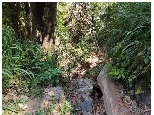
Figure 5d: Seasonal water stream from the upslope towards the railway line in Site No.231
