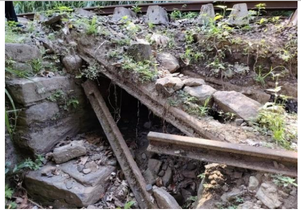
Figure 5b: Seasonal water stream and damaged culvert below the railway line, Site No.231
