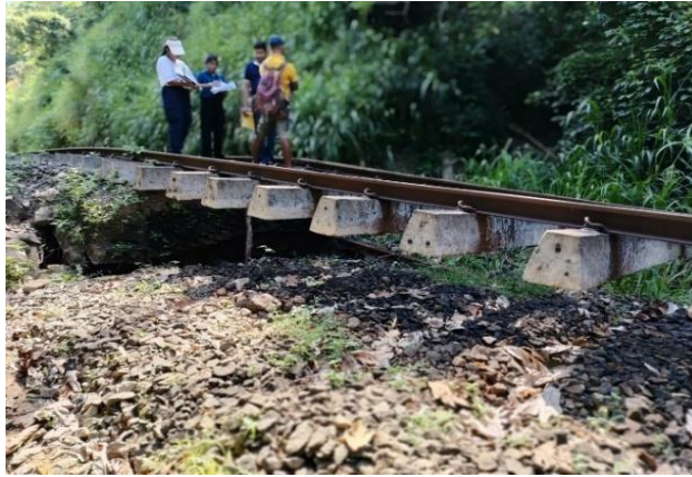
Figure 5a: Vegetation near the washout of the railway line in Site No.231 (CH 60/72)
