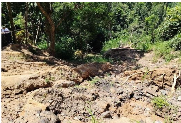
Figure 5e: Vegetation near the landslide of Site No.232, and this area is used as an access road to nearby houses
