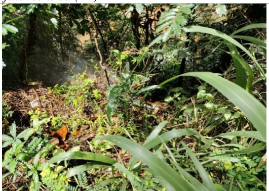
Figure 5s: Broken community water line (L7)
