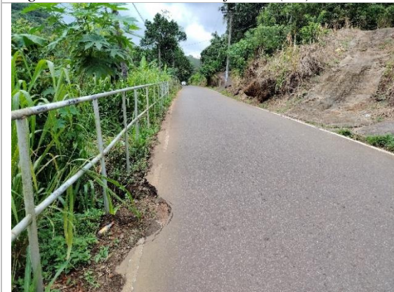
Figure 5x: Damaged Road section due to water flow (L8)
