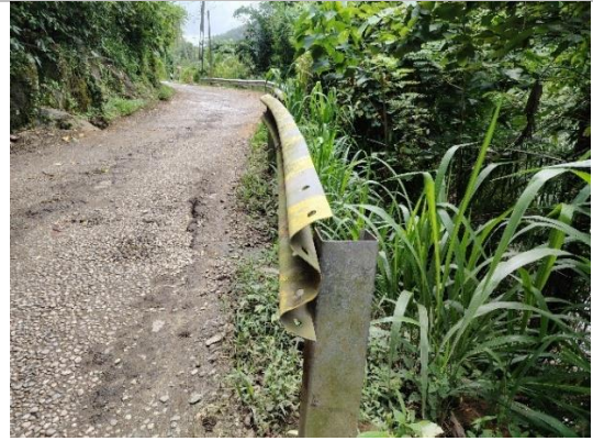
Figure 5o: Damaged Road section with RDA fence (L6)
