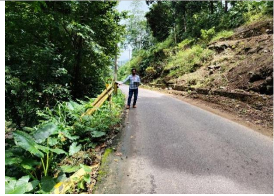
Figure 5d: Broken part of the fence due to landslide (L2)
