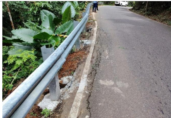
Figure 5h: Cracked Road section in road of RHS (L4)
