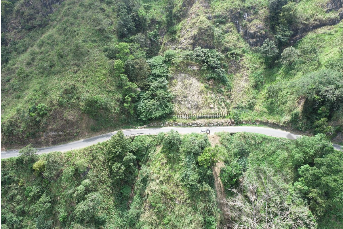
Fig. 3.19 Photograph of the slope with rock debris and down slope
