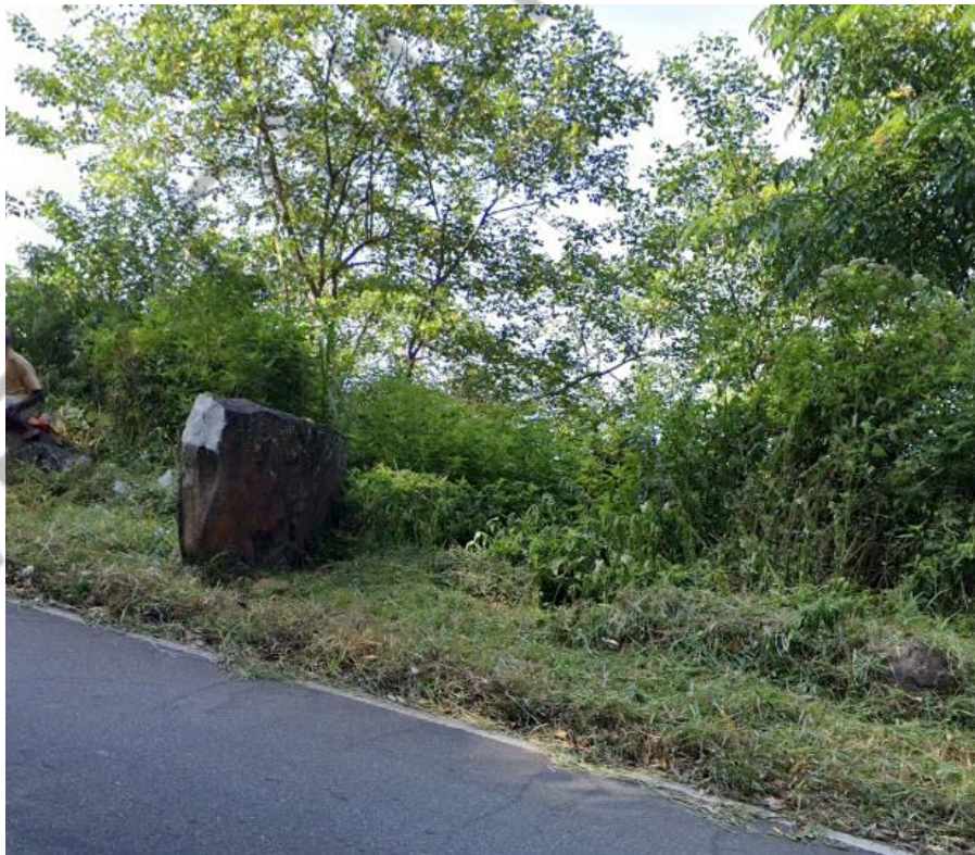
Fig. 3.14 Photograph of the collapsed rock fragments
