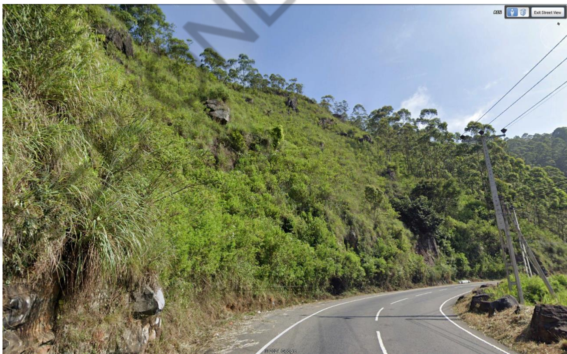
Fig. 3.10 Photograph of the detached rock boulders resting on the slope
