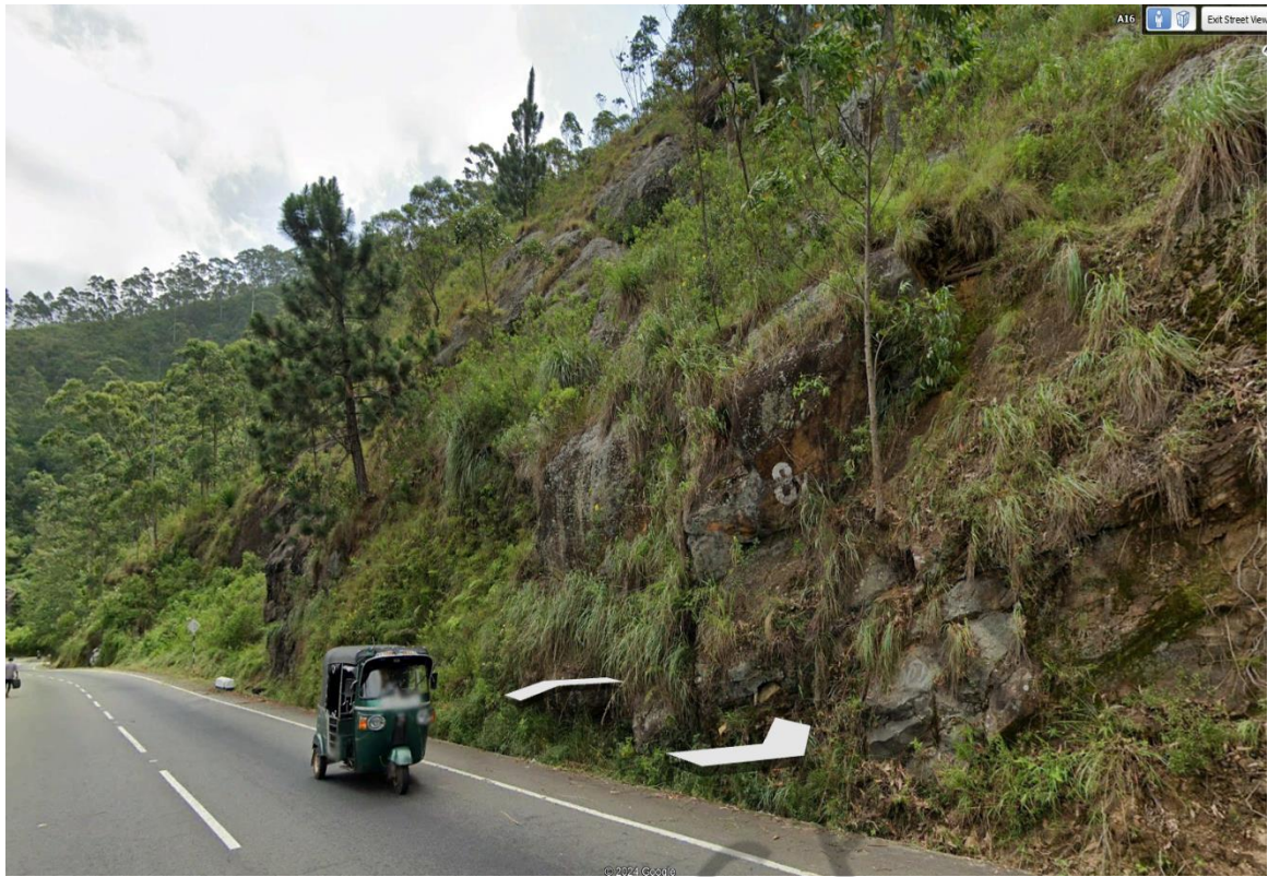
Fig. 3.13 Photograph of the fractured rock slope and detached rock fragments
