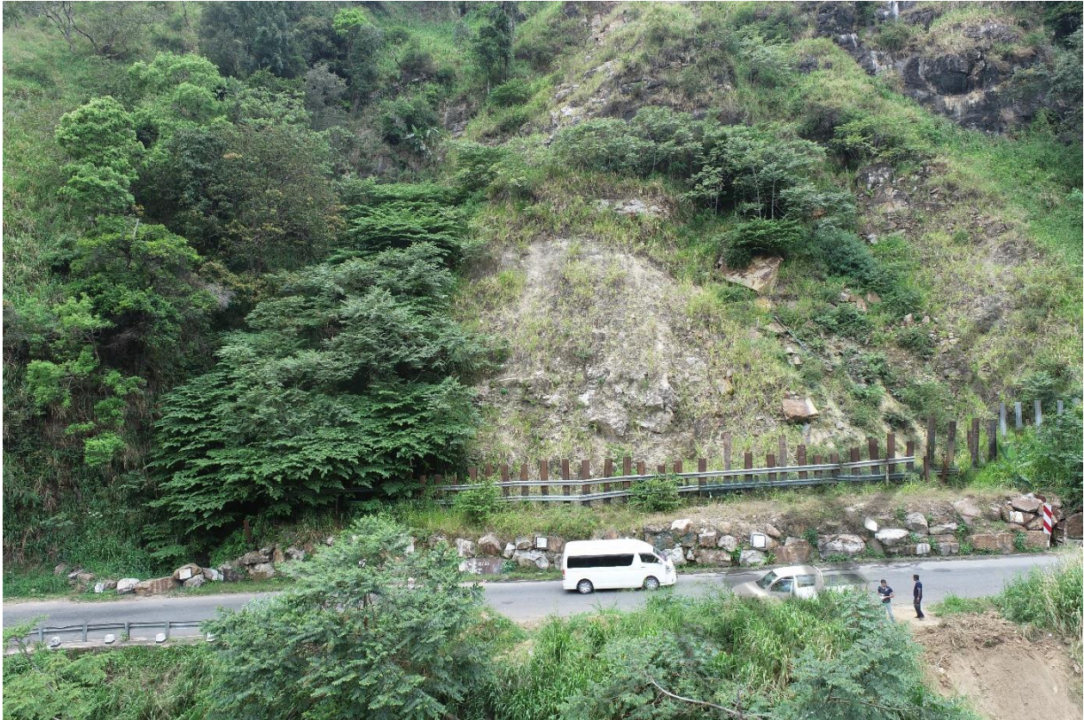
Fig. 3.17 Photograph of the slope with rock debris
