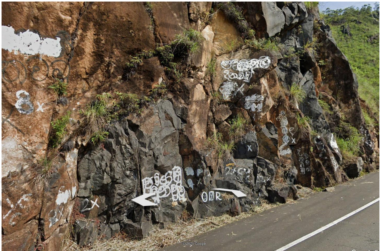
Fig. 3.8 Photograph of the fractured exposed rock in between culvert 5/2 to 5/4
