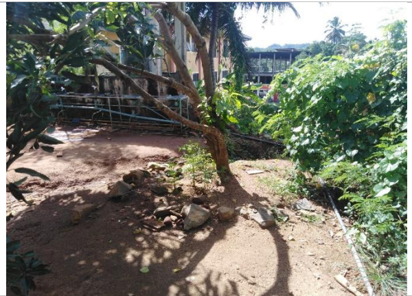
Figure 4f: Slope failure close to washing sink area
