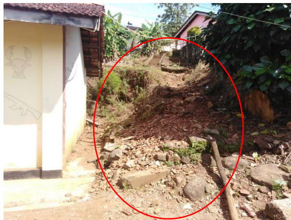
Figure 4g: Slope failure close to Cadet room
