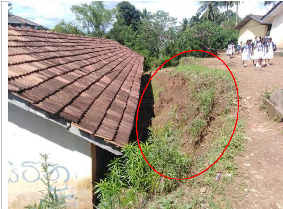
Figure 4e: Cutting failure located upslope of the grade 7 single storied building
