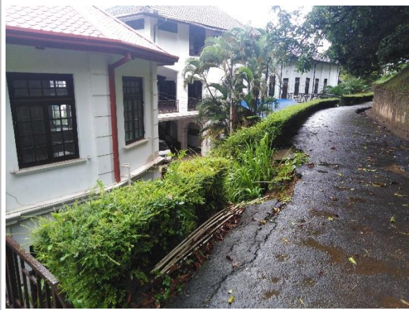
Figure 4e: Failed Road and slope section behind the teacher's sanitary facility and home science laboratory (L5)
