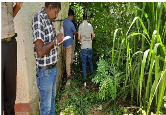
Figure 4I: Unstable land section in between dancing room and newly constructed 4 storied building (L9.)
