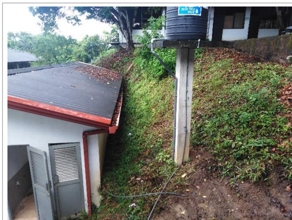
Figure 4a: Slope in front of the grade 12 tec 2 building (behind the sanitary facility) (L1)
